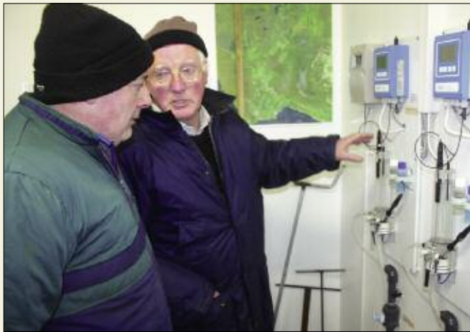
Éamonn McCabe of Bunn GWS discusses the chlorine monitoring system in Meenabool GWS, with local caretaker, Eugene Mooney.
